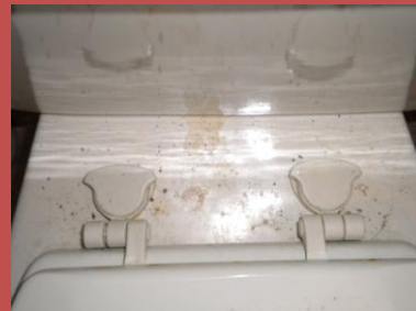
Figure Three: Mold On Toilet
