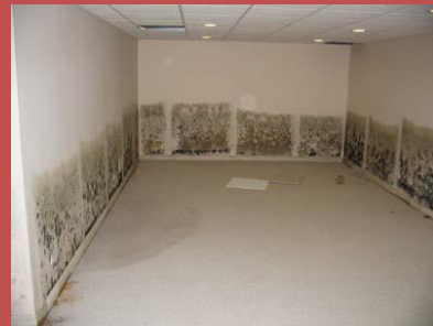
Figure Four: Clean Air and Sciences Mold in Basement
