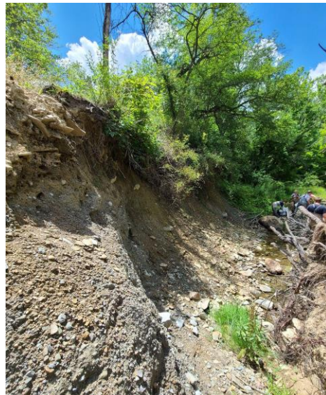
Figure 8: Image of German Run's poorly structured stream bank, which under high flow is heavily eroded.
