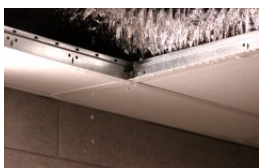
Steam leak evacuates Walker Hall
